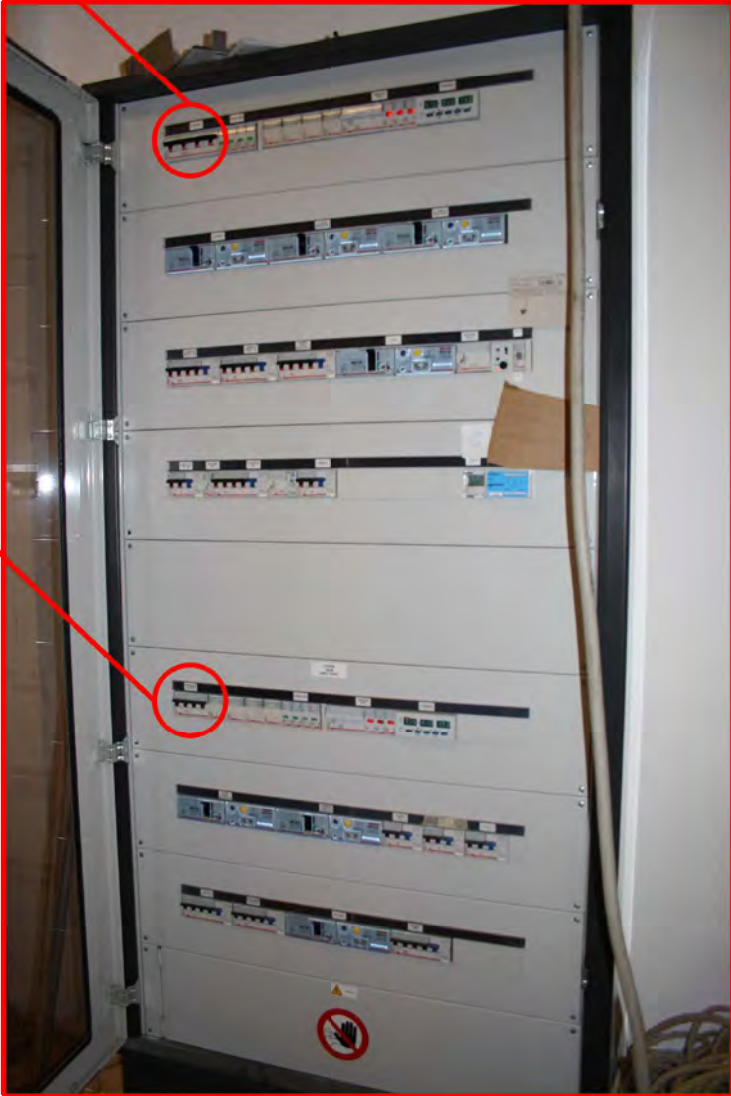
Quadro El. GEN. Auditorium
